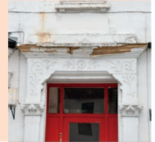
Peeling paint above doorway
