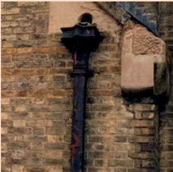
Flaking and rusting downpipe
