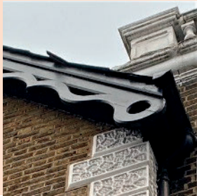
Slipped slate photo after storm damage
