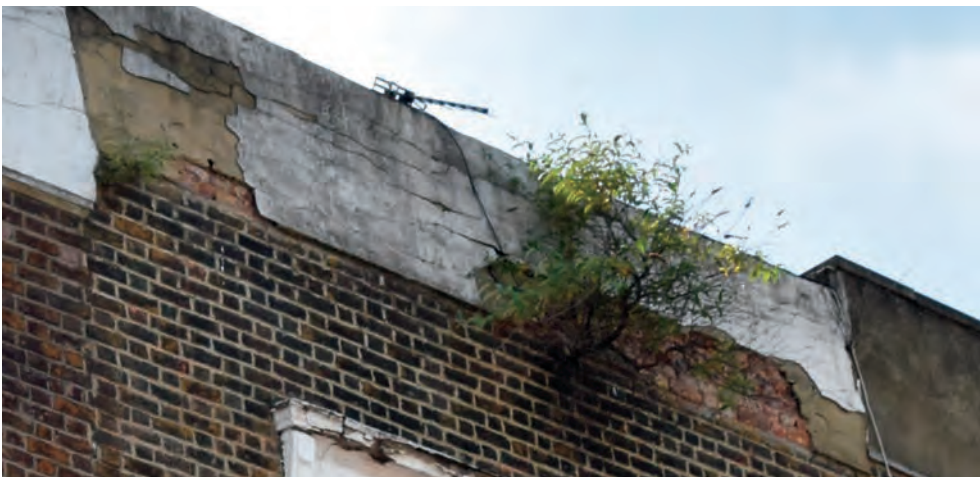
Blocked parapet gutter allowing damp to enter the building
