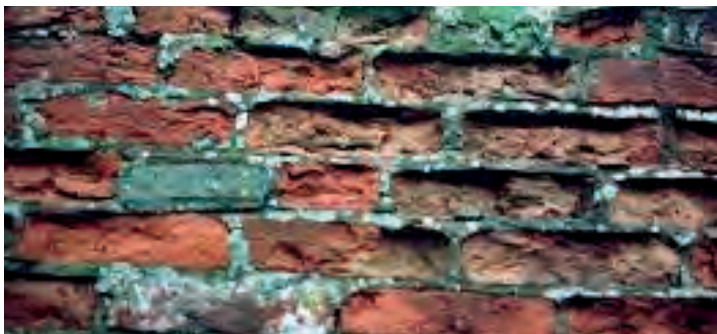
Modern cement pointing to traditional brickwork causing erosion.
