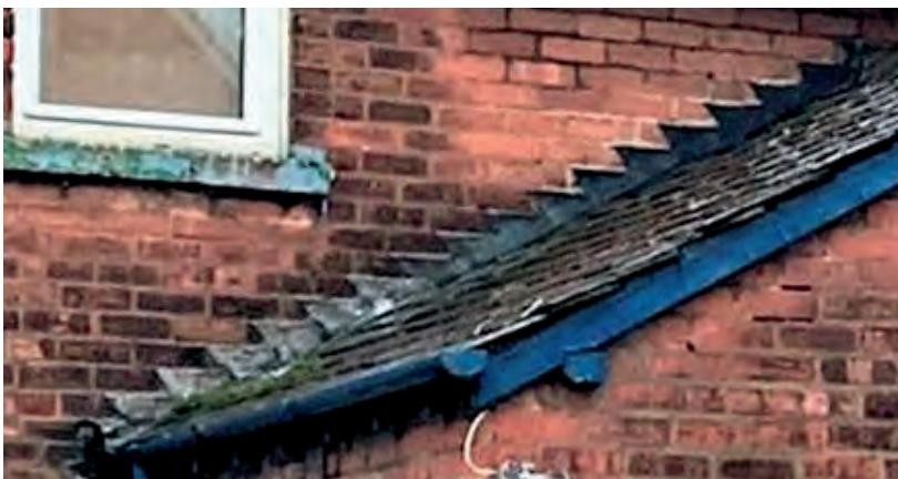
A stepped lead flashing at the abutment of a roof and wall.
