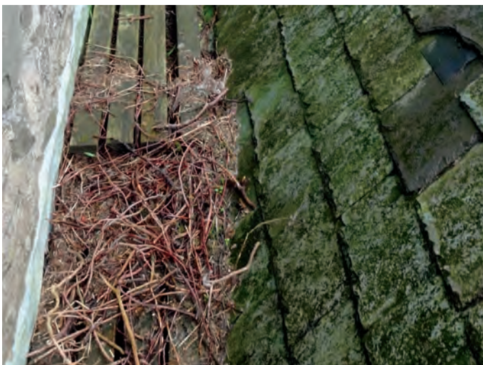
(L) A parapet gutter blocked by nesting material.
