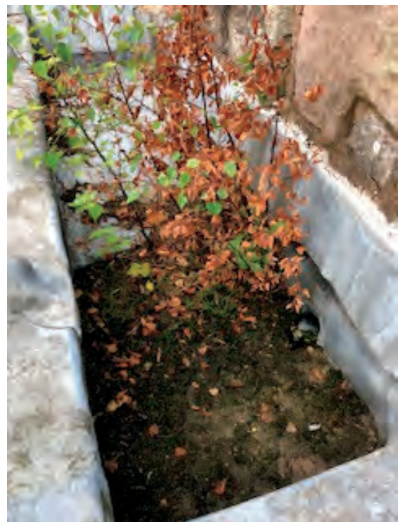
(R) A tree sapling allowed to grow in a parapet gutter.
