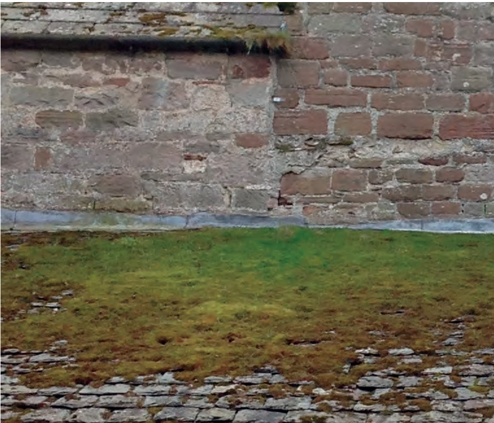
Excessive moss growth on roofs.
