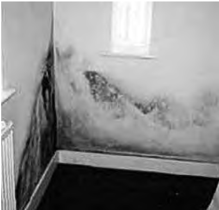
Mould growth, often an indication of condensation
