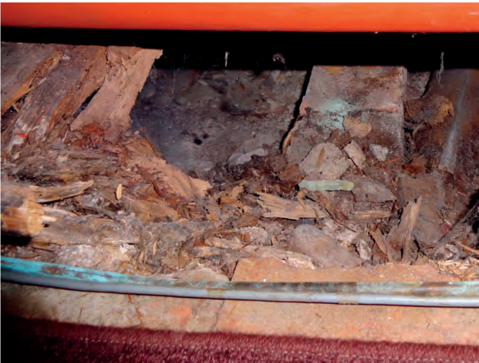
Dry rot caused by lack of ventilation to the floor void
