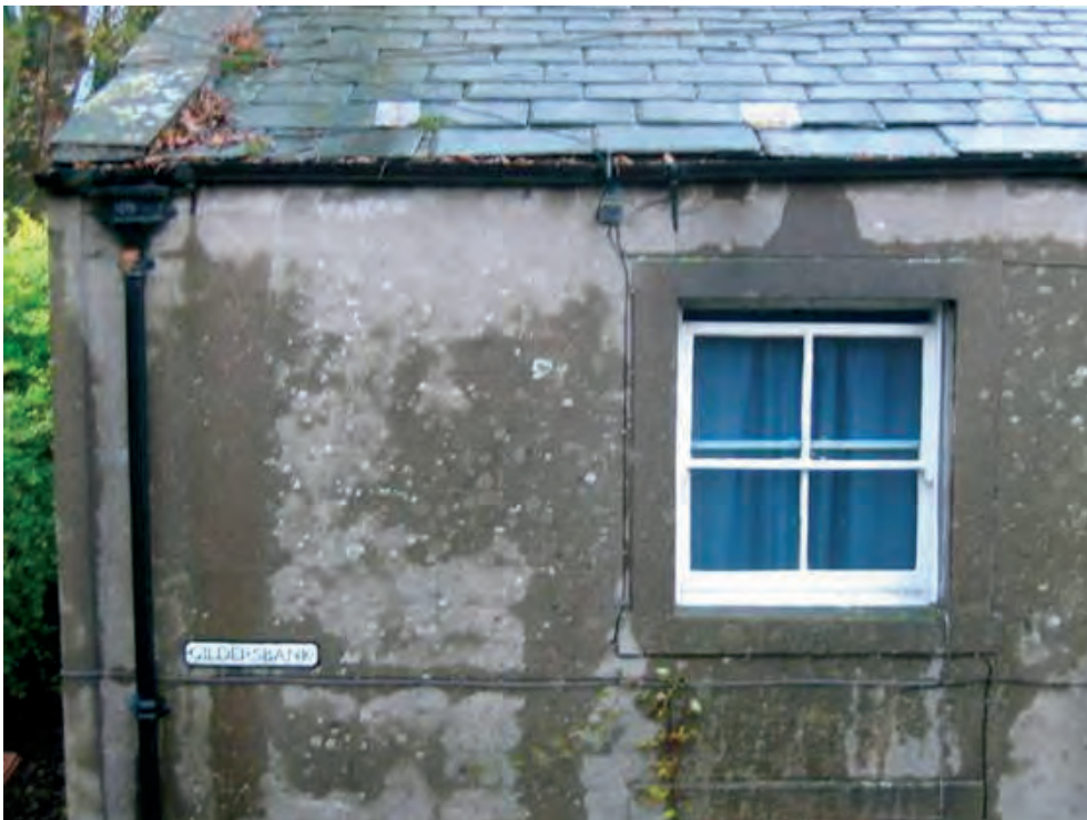
Location of blocked gutter evident after heavy rain.
