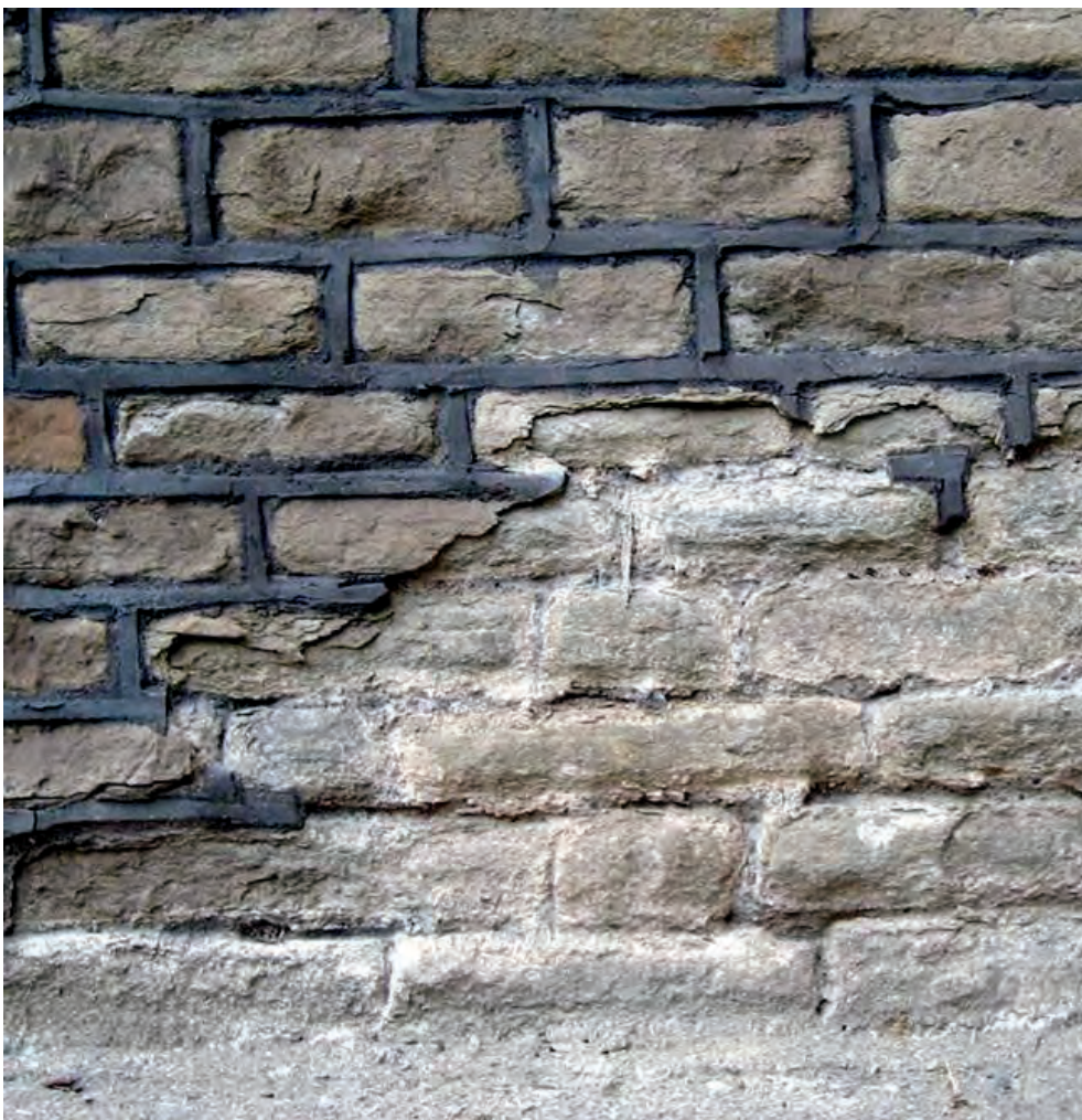
Erosion to soft stonework caused by modern cement pointing
