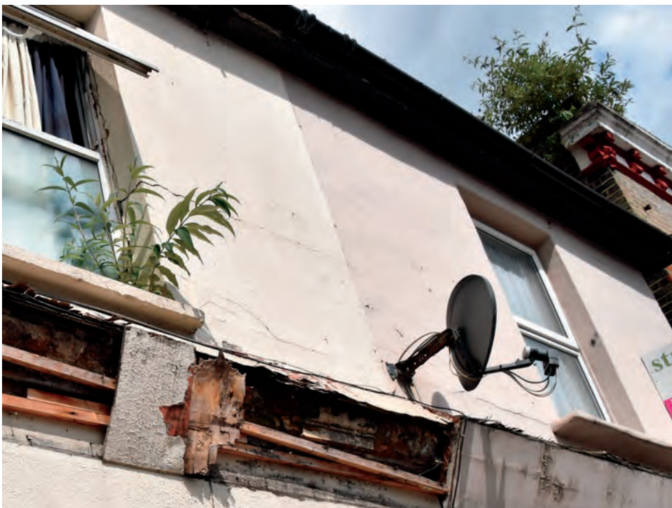
Decay caused by lack of maintenance.
