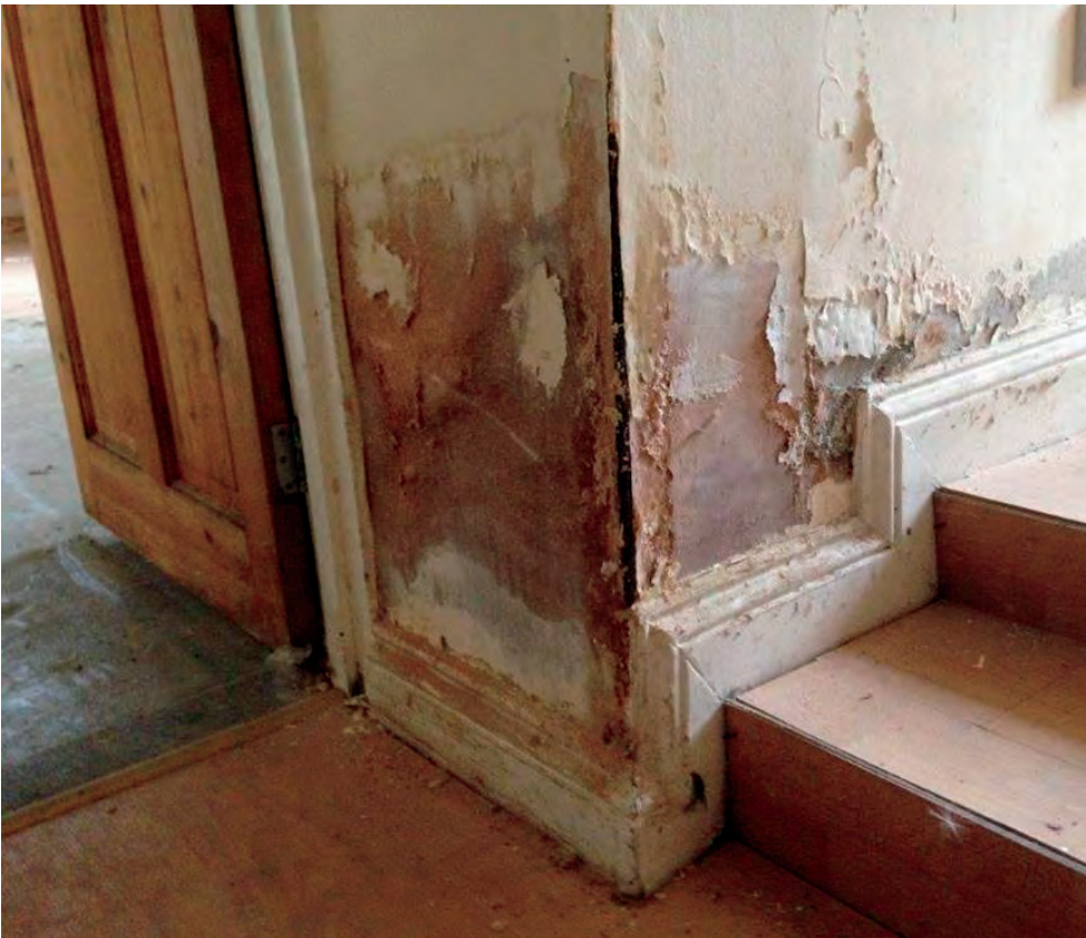
Rising damp to the base of the wall
