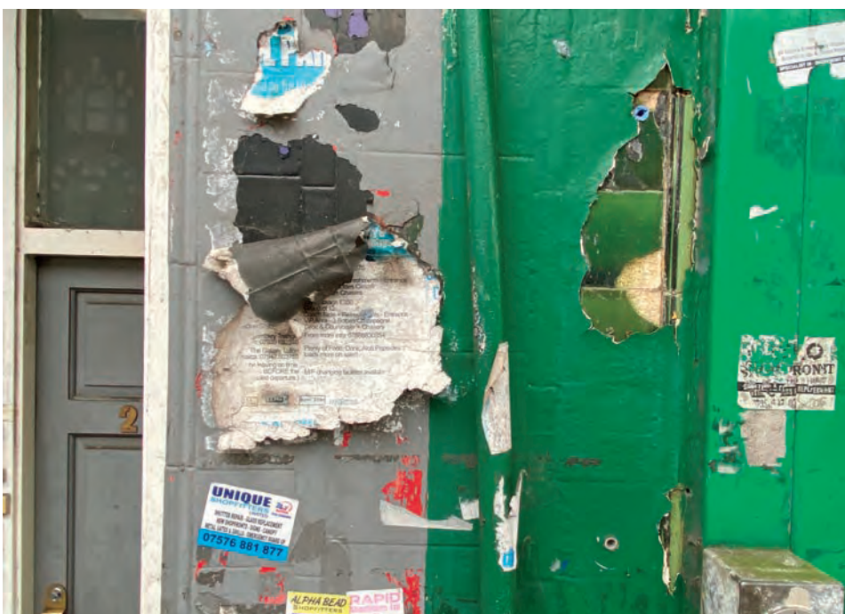
Blistering and failure of an impervious external paint finish.
